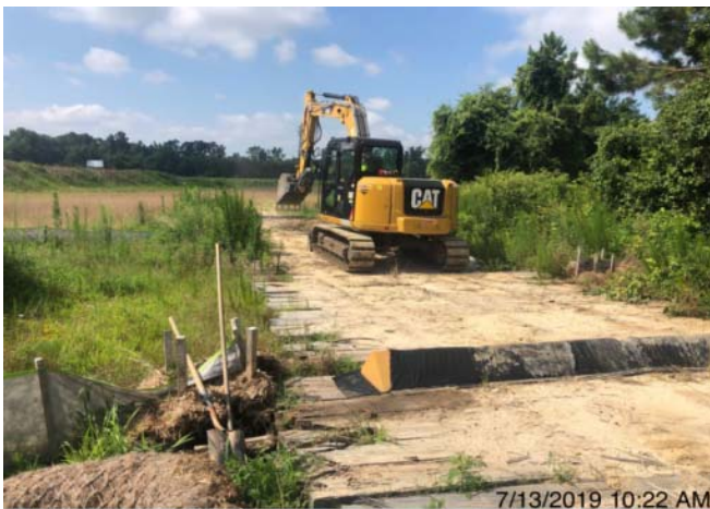
Spread 8 – ECD Maintenance
