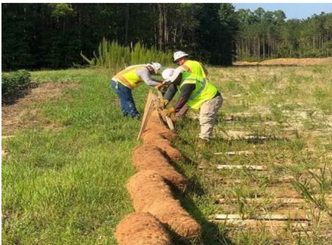
Spread 8 – ECD maintenance
